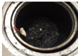
Inside the compressor
