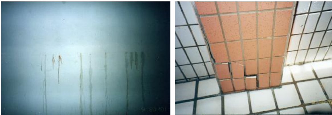
Figure 7: Water leaking due to horizontal crack in a basement wall (left) and a column (right)
