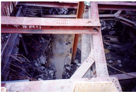
Figure 6: Groundwater flooding on finished surface
