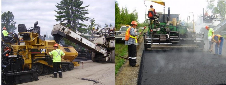
Figure 8: HL8 binder course paving. Figure 9: Echelon paving and material transfer vehicle were employed for surface paving and temperatures were checked constantly.
