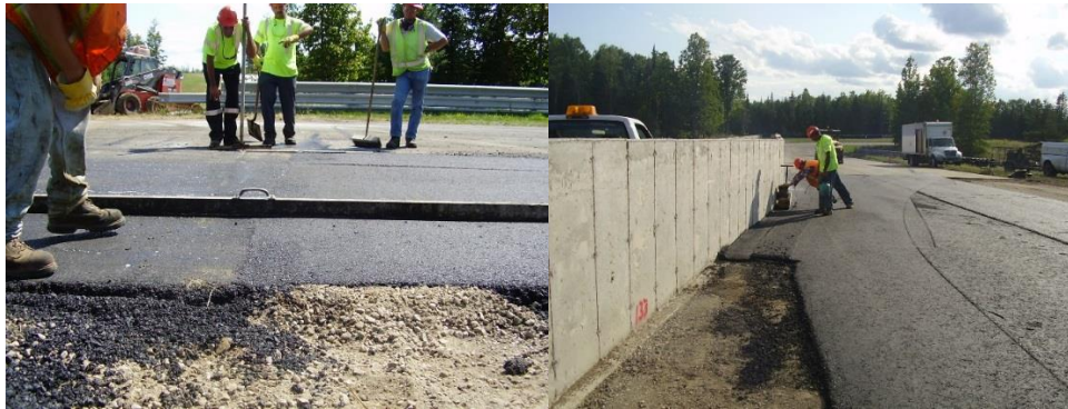
Figure 12: Checking smoothness in a horizontal joint. Figure 13: Compaction in the edge by portable tamper plate.
