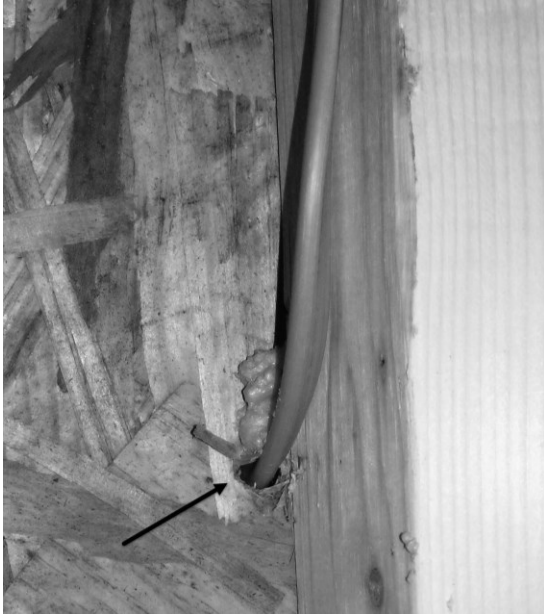
Figure 1. Poor Foam Air Sealing
