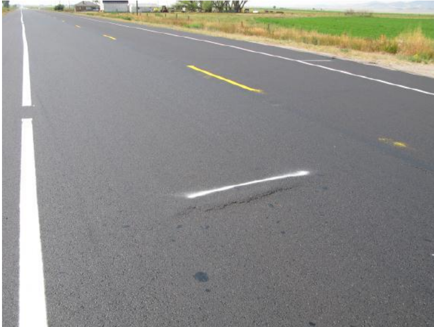
Figure 1: Transverse Bump in New Asphalt Overlay Placed Over Crack Sealant
