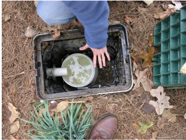
Figure 7a: PC Leachate collection reservoir
