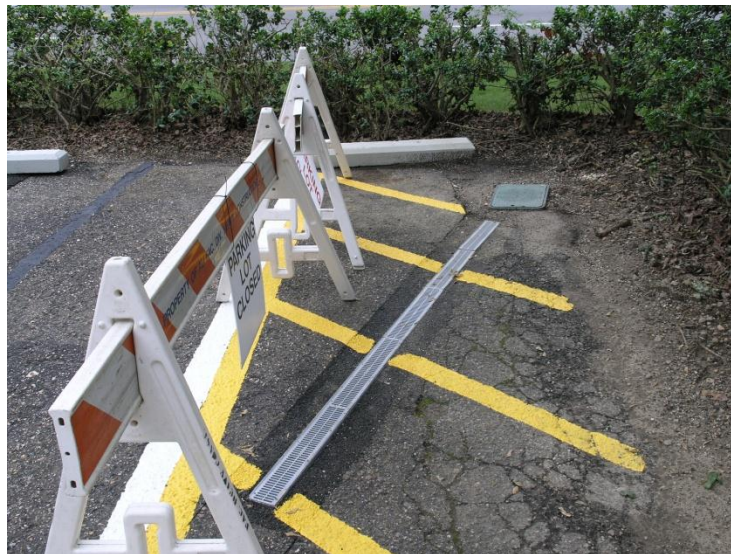
Figure 6: Drain for collection of surface runoff from asphalt pavement
