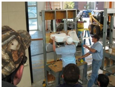
Figure 4: A plumber and his helper demonstrate how to install fixtures in Laboratory #4
